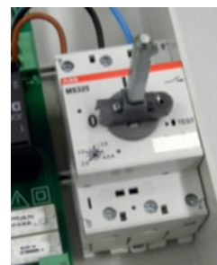
Motor protection breaker switch Motor protection
