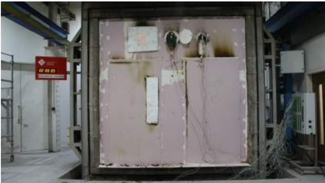
Figure 30 - The unexposed surface of the test construction after a test duration of 120 minutes
